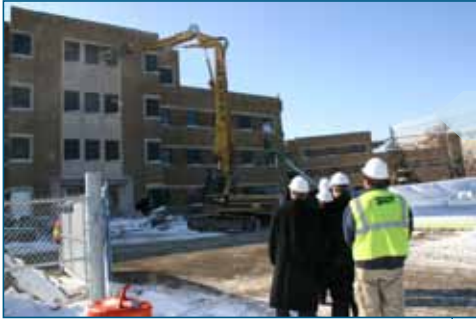
Excavators demolish part of the vacant former Larue D. Carter Psychiatric Hospital as Mayor Gregory Ballard, City-County Councillor Michael McQuillen and Wishard project and construction leadership look on.
